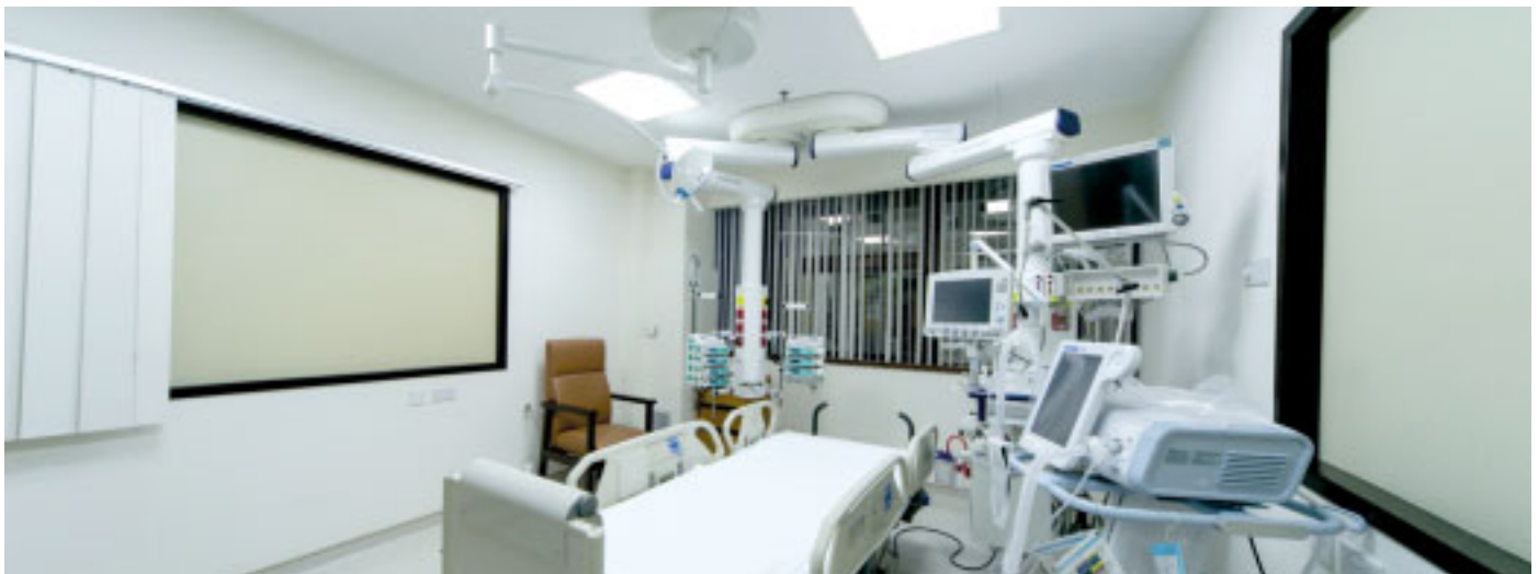
Gleneagles Hospital Singapore's LED lighting plan extends to its operating theatres.
